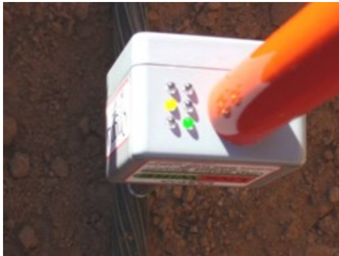
Dead or De-energized ( Green ) Indication
