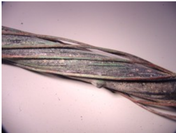
Severely Corroded Semi-Conductor and Concentric
